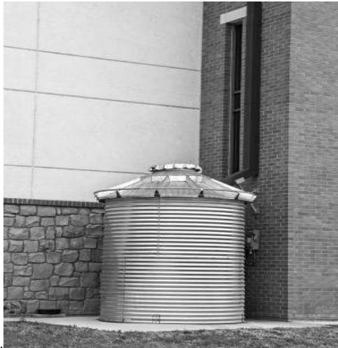
Figure 1 Rain Water Storage Tank is connected to Ground Water Recharge
